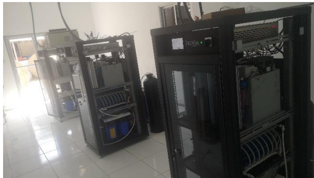
HPGen production center at Agrolíbano, composed of three HPGen A-Series systems.
